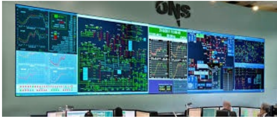
Figure 1 – Room of Electric Power Control and Operations Center Source: ONS, 2014.
